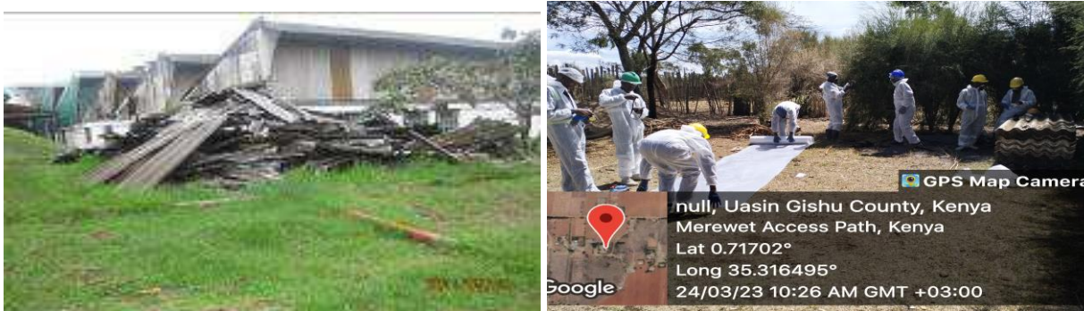
Poorly managed asbestos: A licensed transporter preparing to transport the removed asbestos waste for disposal
