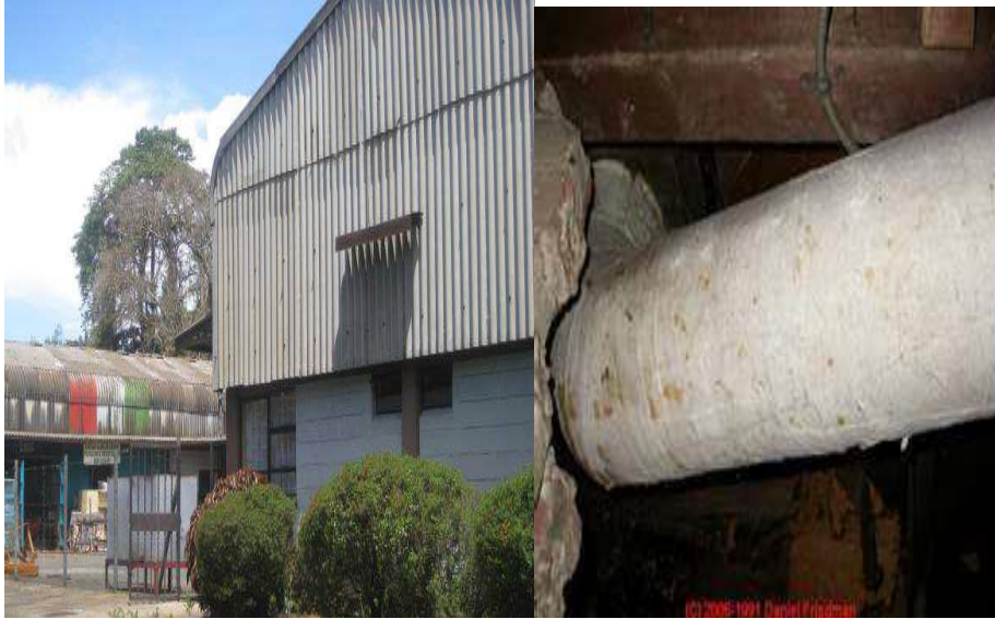
A photo of asbestos used as roofing material and boiler insulation
