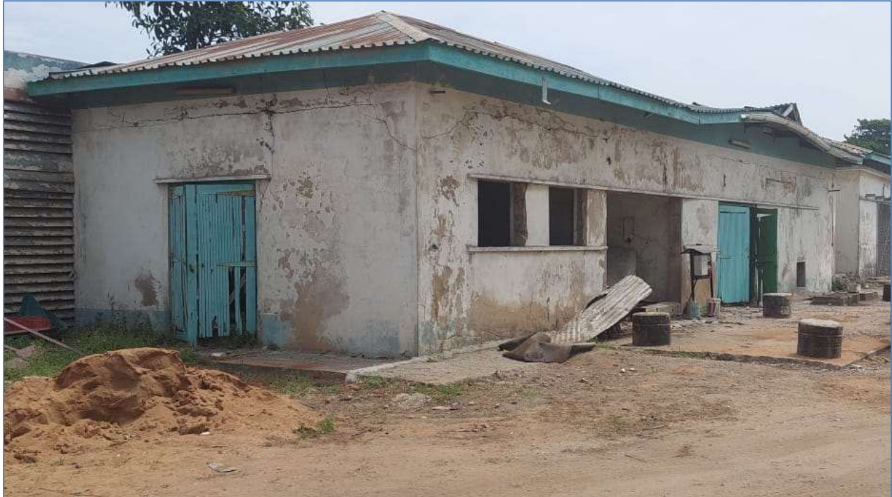
Figure 2: A section of the dilapidated warehouses at the proposed project site which were previously used by Kenya Meat Commission (Source: site visit, January 2022).
