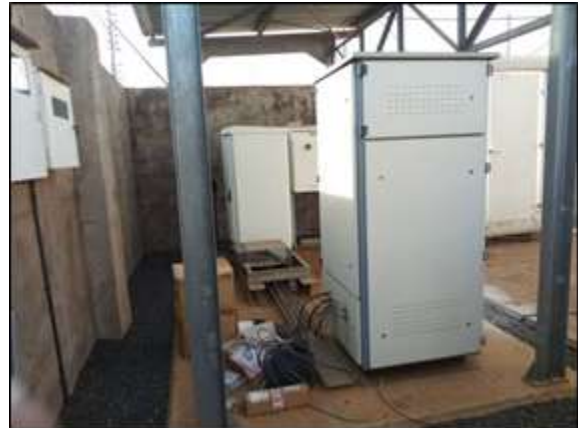
Plate 1: Typical Cabinet Structure
