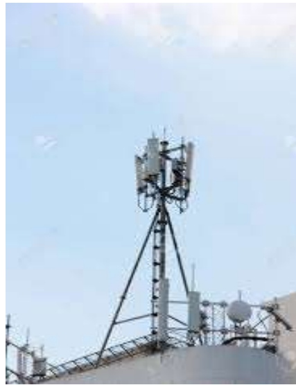
Plate 1: Photo of a Typical Rooftop BTS.
