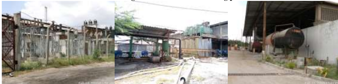
Plate 2: Support facilities of the steel mill i.e. 33KV sub-station, water cooling system & bulk IDO storage
