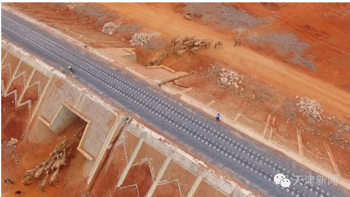
Plate 6- 20: Structure of a wildlife and livestock underpass culvert in the SGR Phase I project
