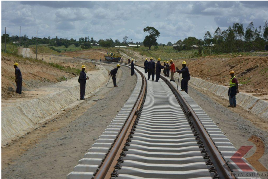
Plate 2- 1: Shows the drainage system used in SGR-I
