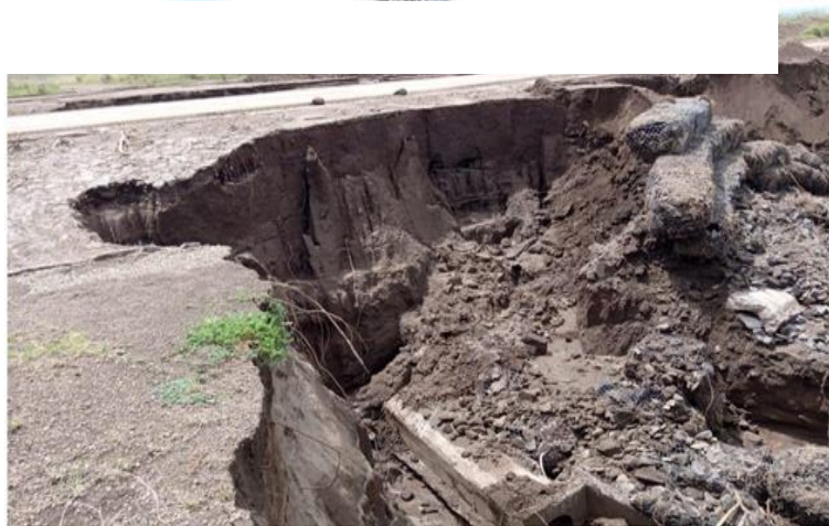
Figure 11: Previous Impacts from floods in the adjacent areas
