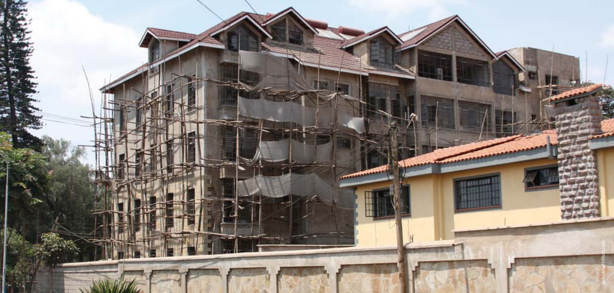
A building under construction in Nairobi. Construction's contribution to the real GDP grew from 49.1 billion in 2009 to 51.4 billion in 2010.
