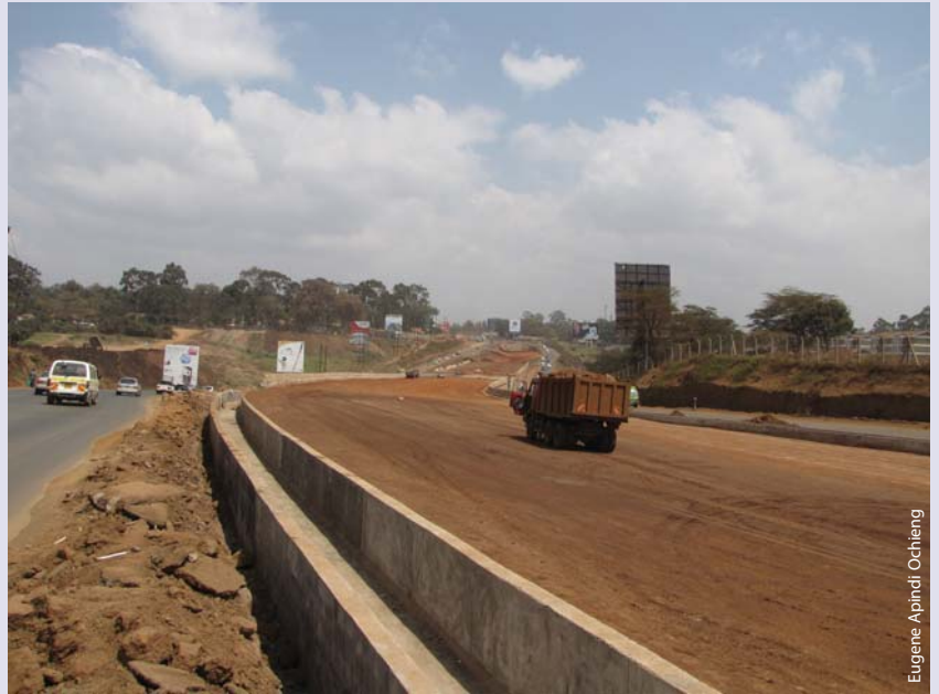
Construction of the Superhighway and drainage works at the Utalii College/ National Youth Service (NYS) area.
