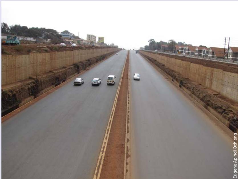
A completed section of the Thika Superhighway express lanes, close to Garden Estate.
