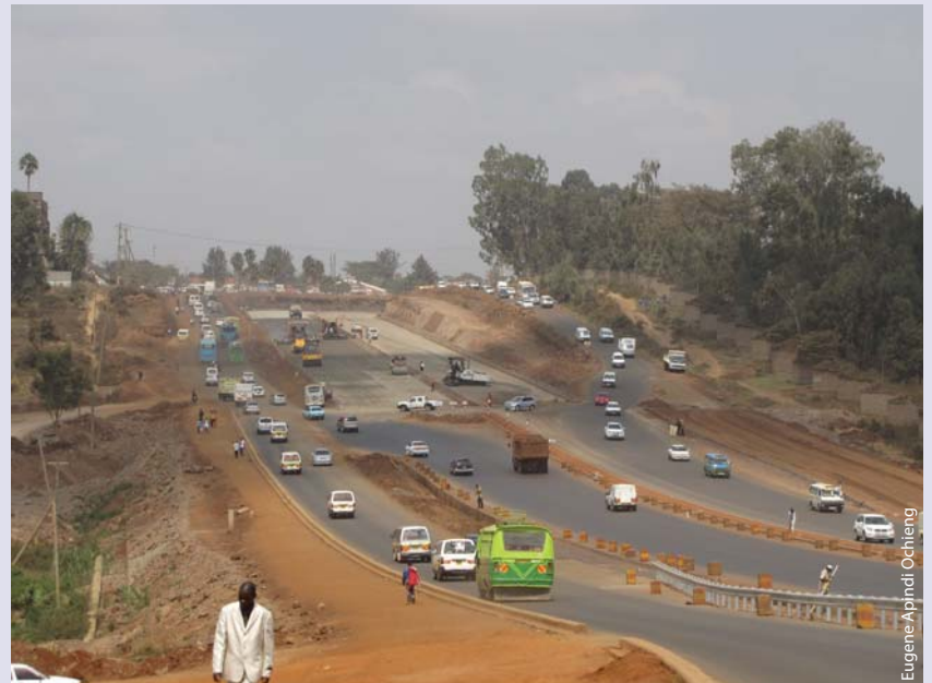
On-going construction on a stretch of the Thika Superhighway approaching the GSU headquarters. The large roundabout that existed in front of the GSU headquarters has been done away with.
