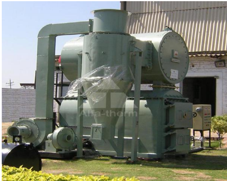
Plate 1: Example of assembled Incinerator
