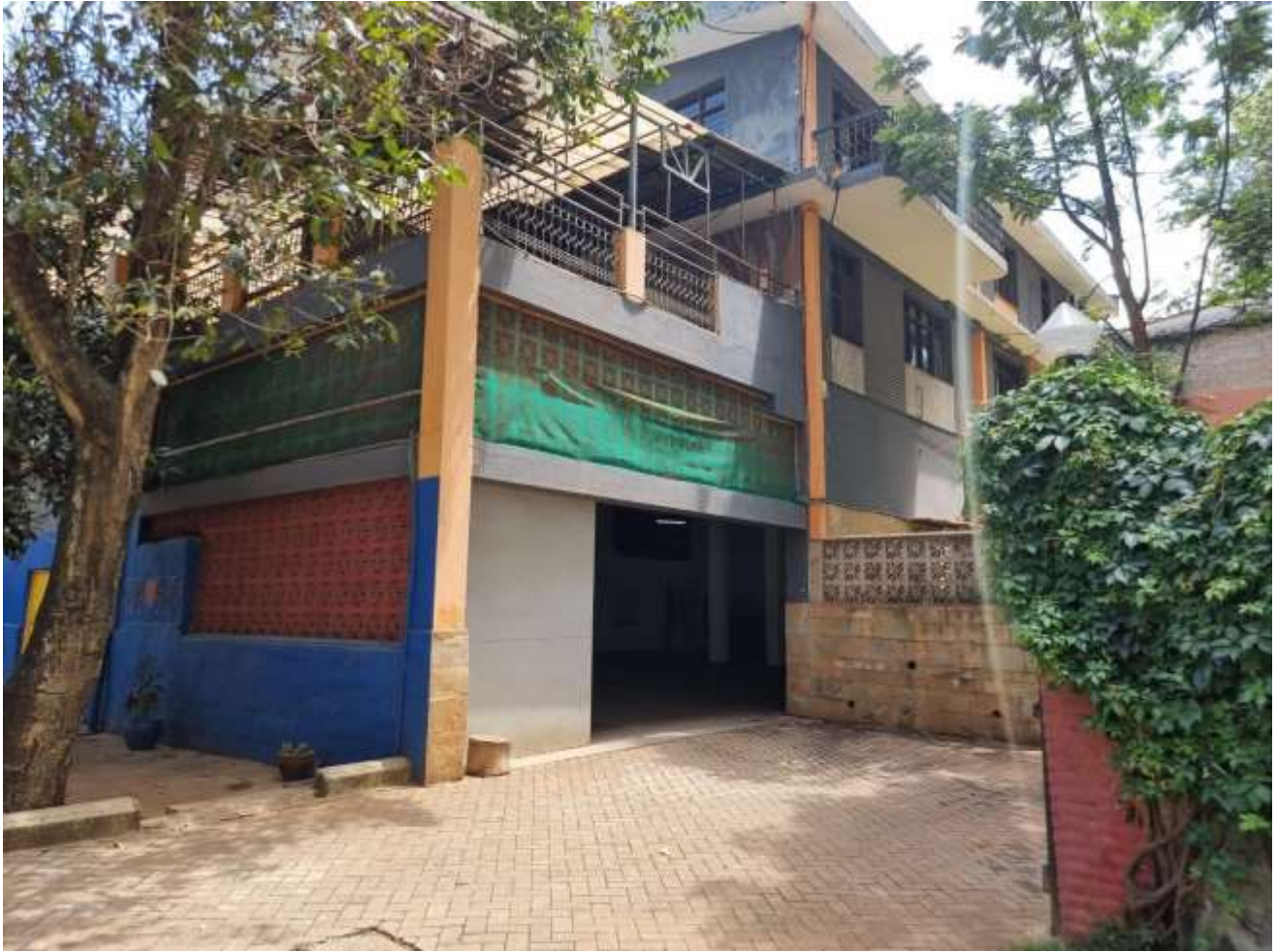
Photo 9: Showing part of the Existing building on site that will be demolished to pave way for the proposed project.
