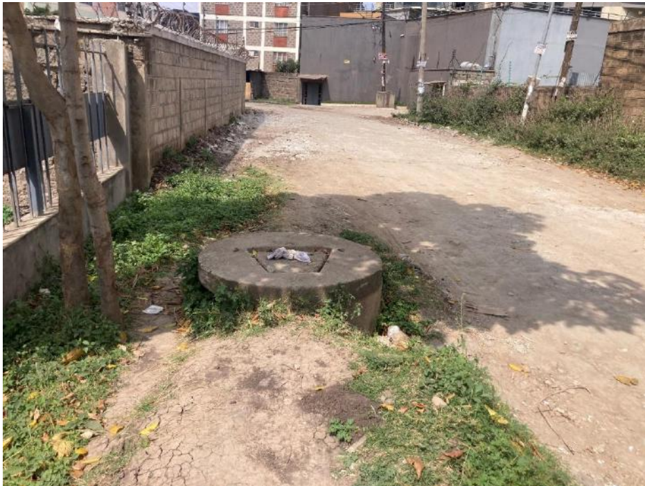
Plate 7: Sewer line manhole on the backside for the project site (adjacent to the Jehovah Witness Church)
