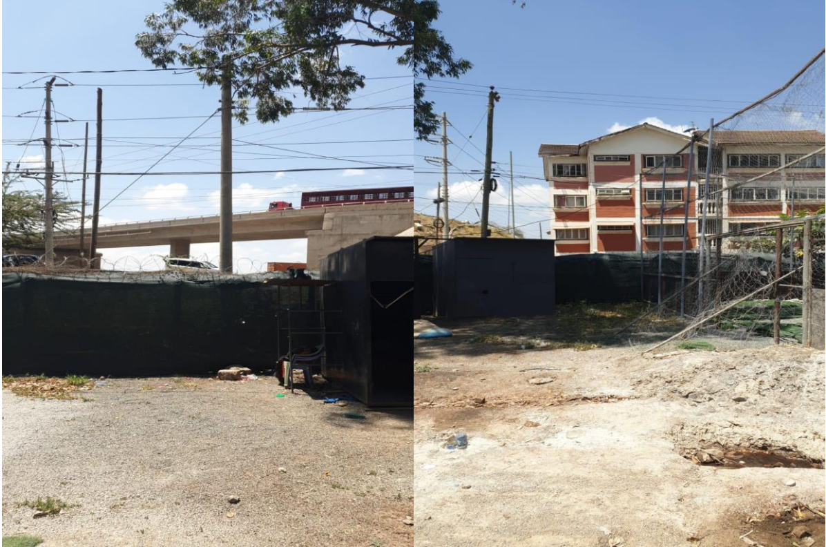
Plate 1: Section of project site fenced off for a mini football pitch on site and some evidence of geotechnical investigations
