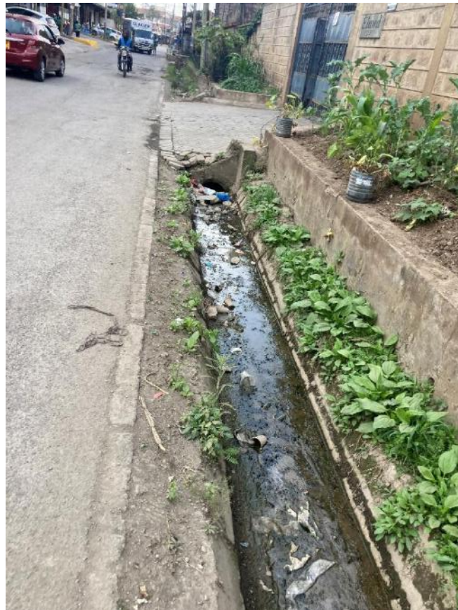
Plate 8: Storm drain along access road leading to Eland Court & Highway Estate South C.
