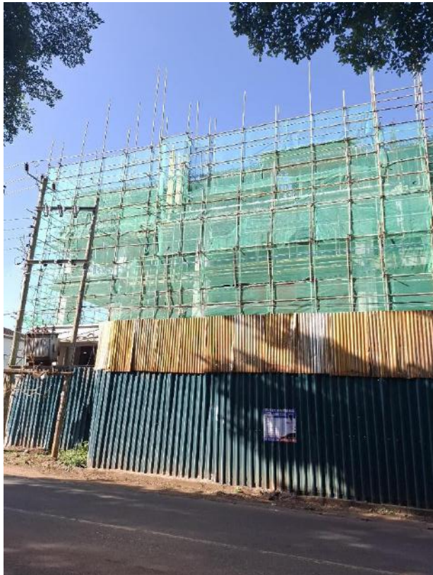
Figure 3. A highrise 18-floor building under construction along Rhapta Road about 50 metres from the project site
