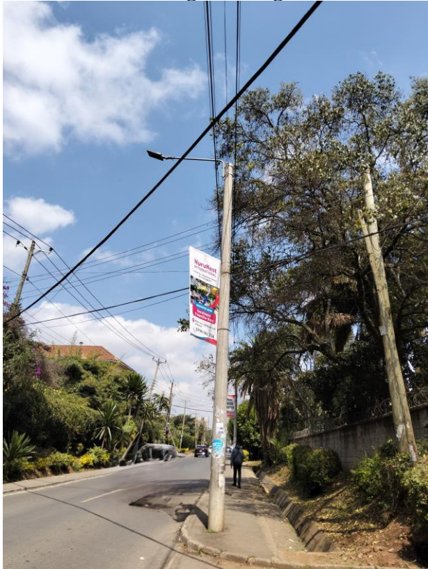
Plate 2. 7: Street Lights along Riara Road
