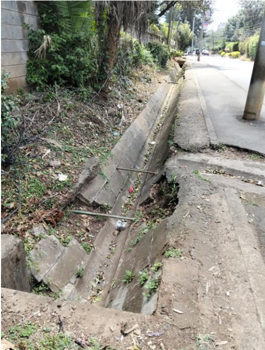
Plate 2. 6: Open Drains along Riara Road
