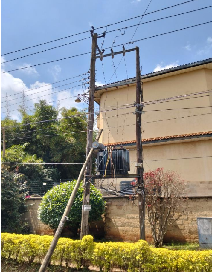
Plate 2. 5: Electricity Transformer along the Riara Road
