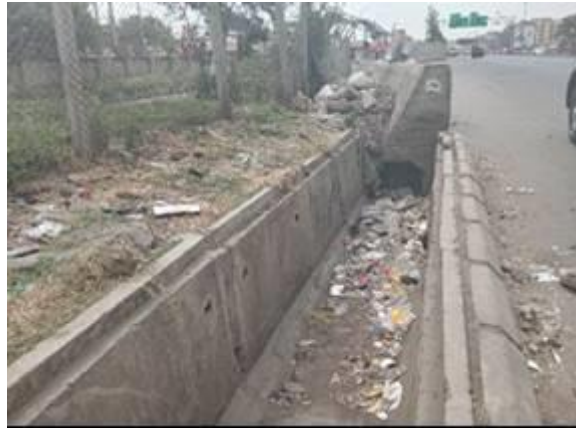
Plate 81: Blocked Stormwater Drain along the Project Road at Pipeline Section
