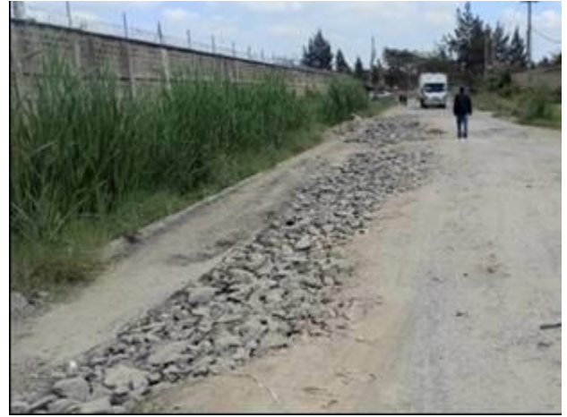
Plate 49: Deteriorated Section of the Project Road
