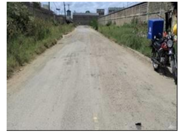
Plate 53: No Provision of Pedestrian Footpaths along the Project Road
