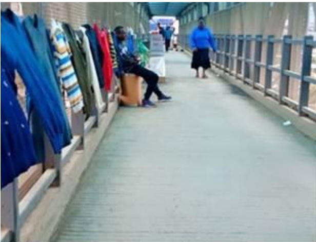
Plate 10: Encroachment at a Pedestrian Footbridge hindering proper use
