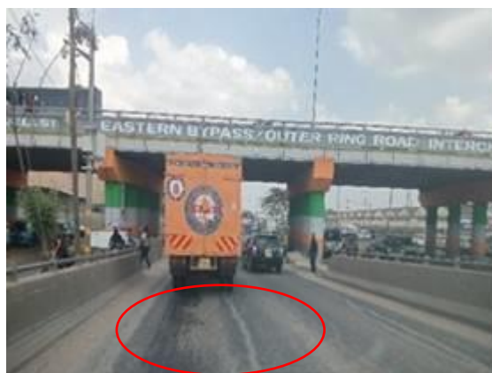
Plate 79: Pavement Rutting along the Project Road at Taj-Mall Roundabout
