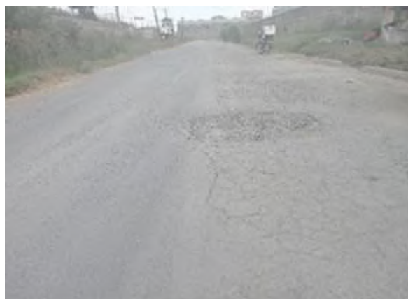
Plate 78: Pothole along Access to the Proposed Depot at City Cabanas
