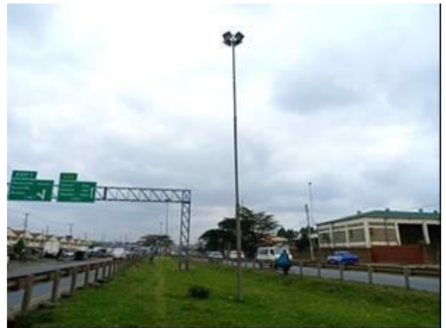
Plate 15: Street lighting Installed along the Median
