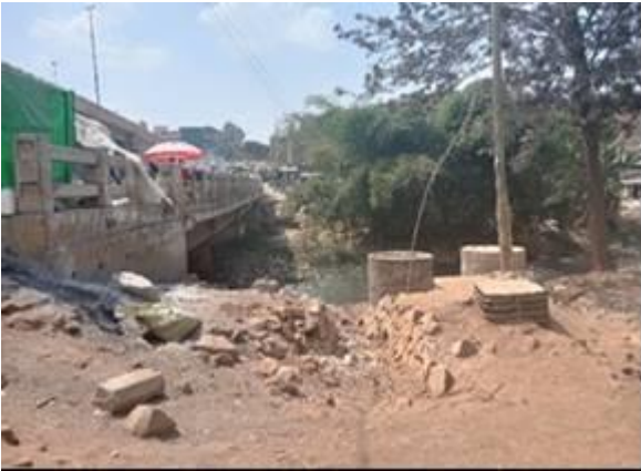
Plate 82: Eroded Section of Mathare River Bank along Project Road at Kariobang Underpass
