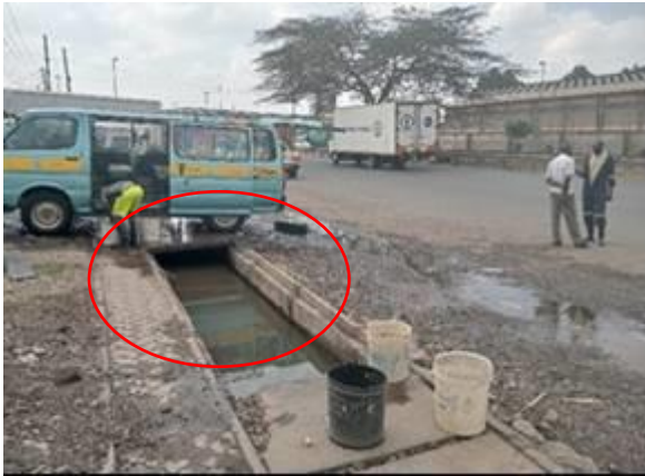
Plate 80: Blocked Drainage along the Project Road, Airport Stage Section
