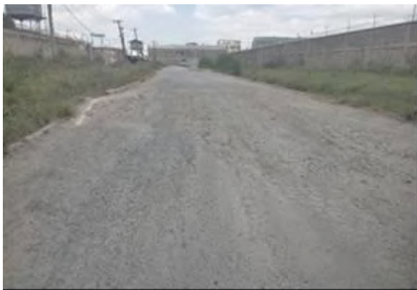
Plate 76: Damaged Road Pavement along Access to the Proposed Depot, City Cabanas
