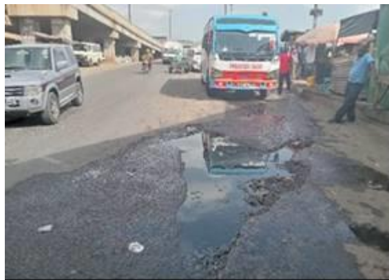
Plate 77: Pothole along the Proposed Project Road, Taj-Mall Bus Station
