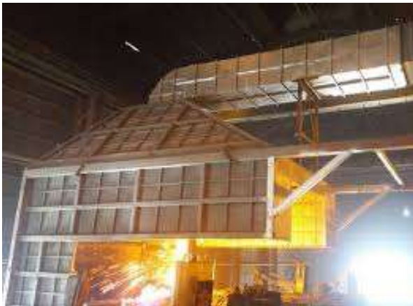
Figure 1: Dog-House Furnace Hood
