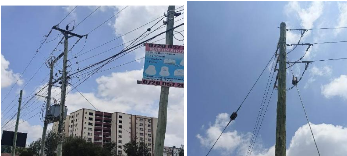
Plate 5: KPLC transformer and Power lines in the project area
