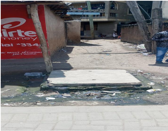
Figure 6.2: An overflowing sewer man hole within the settlement
