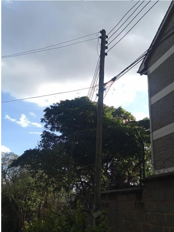
Plate 4. 6: Electricity Lines along the Access Road
