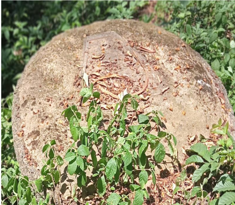
Plate 4. 5: Sewer Manhole within the Site
