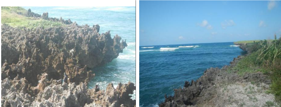
Plate 2 considerably eroded sharp and rugged limestone cliffs at the shoreline of MCL Vipingo site
