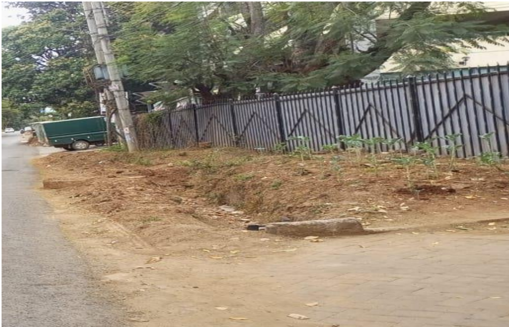
Photo 4: Showing drainage system, along Mogotio road, Westlands area
