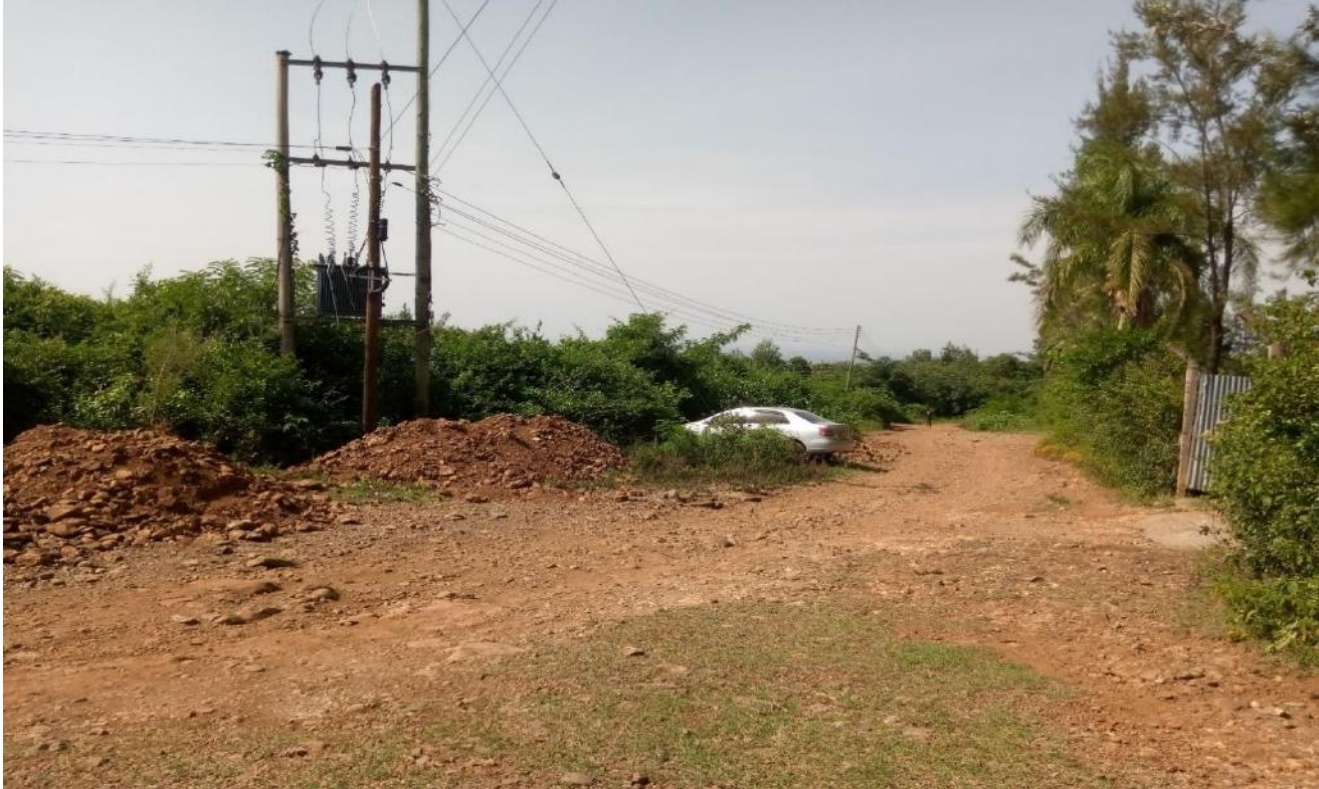
Image: KPLC transformer opposite the site entrance.
