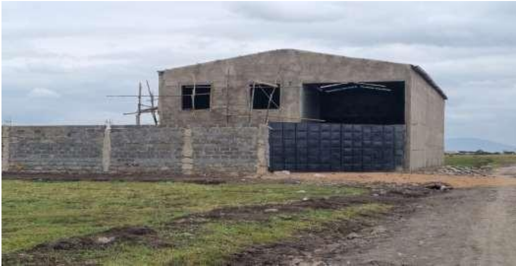
Existing Godown for the Installation of Machinery and Equipment for the proposed steel processing plant
