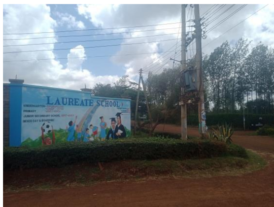
Plate 8: An existing transformer near the proposed site. Source Field Survey
