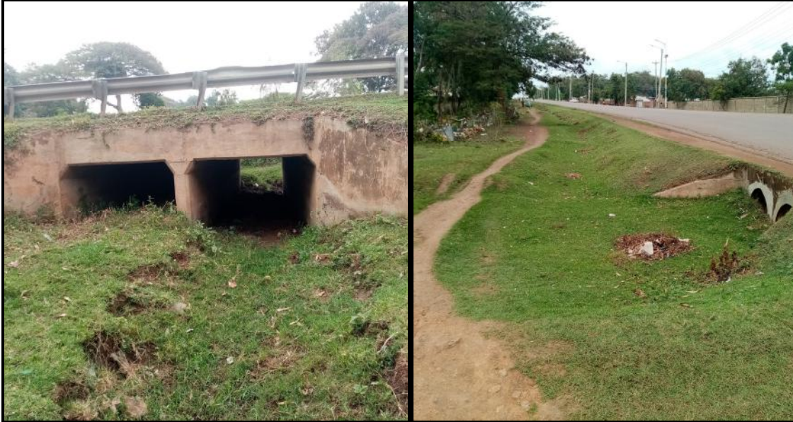
Figure 14: Existing storm water drainage with the vicinity of the proposed project site.
