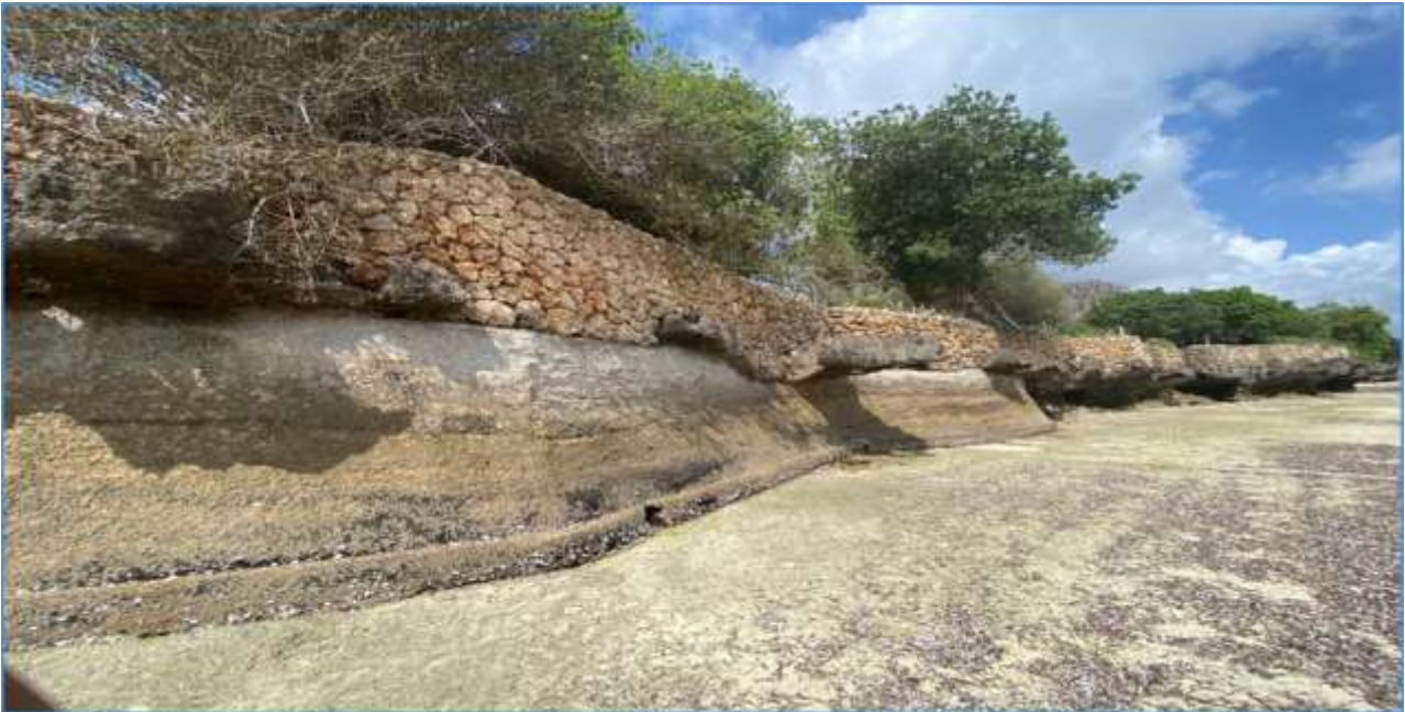
Figure 6: A section of an existing seawall along the shoreline, adjacent to the project site (Source: Site visit, November 2022)
