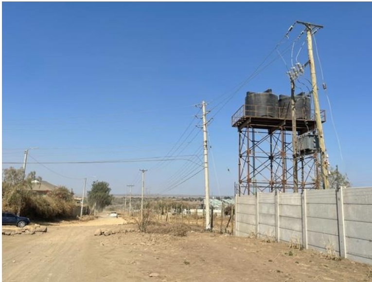
Photo 6: KPLC connection at the project site
