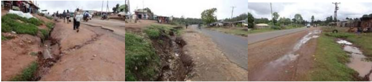
Figure 4-3: Drainage along the road Compromised Roadside Drainage (Typical of KM0+000 – Km55)
