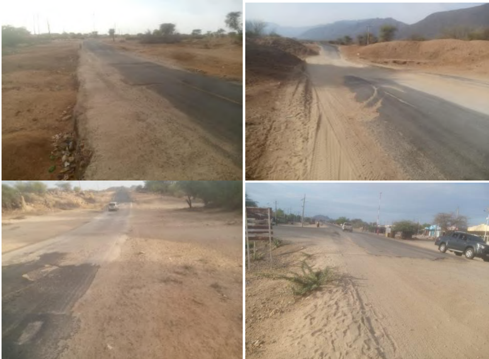
Plate 2 Showing condition of the pavement of various sections of the project road.
