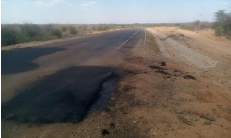
Plate 1: Showing a paved section under the stage construction methodology with numerous sections requiring frequent patching
