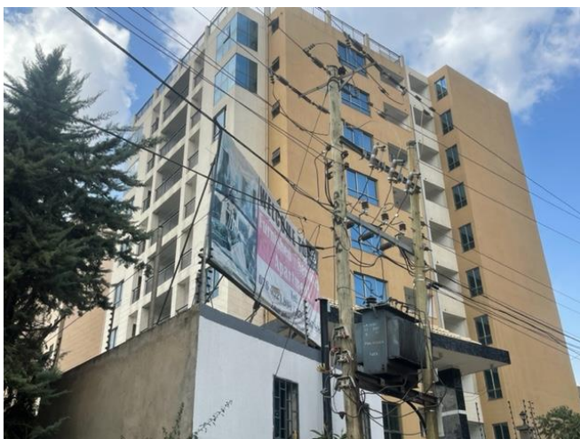
Photo 8: KPLC power line connection along the project site
