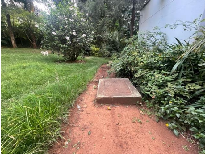
Photo 7: A connection Nairobi City Water & Sewerage Company Sewer-line along the site
