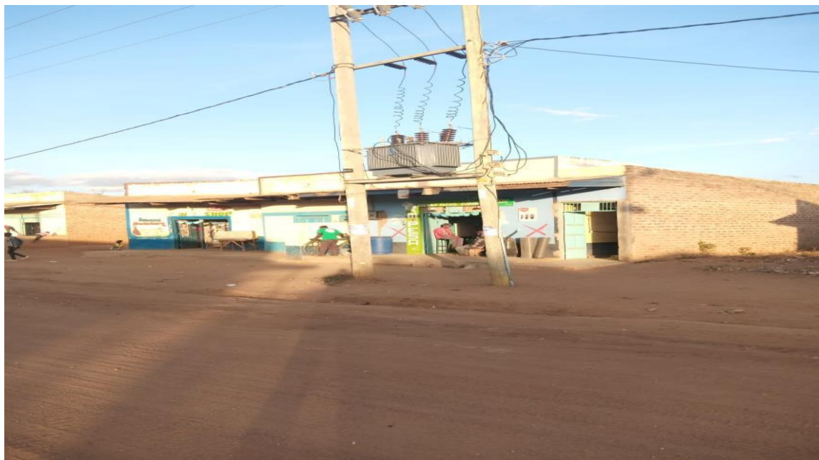
Plate 8 Power lines along the proposed project route
