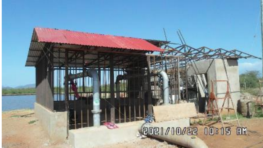
Figure 2-10: Main and Slave Pump at the site
