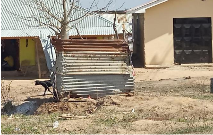
Figure 8: A dilapidated Pit-latrine within Makamini Trading Centre (Source: Field Survey, 2021)
