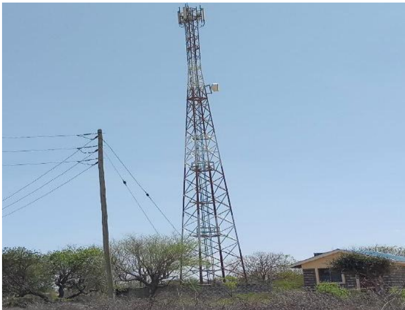
Figure 13: Base Transceiver Station at Makamini Trading Centre (Source: Field Survey, 2021)
