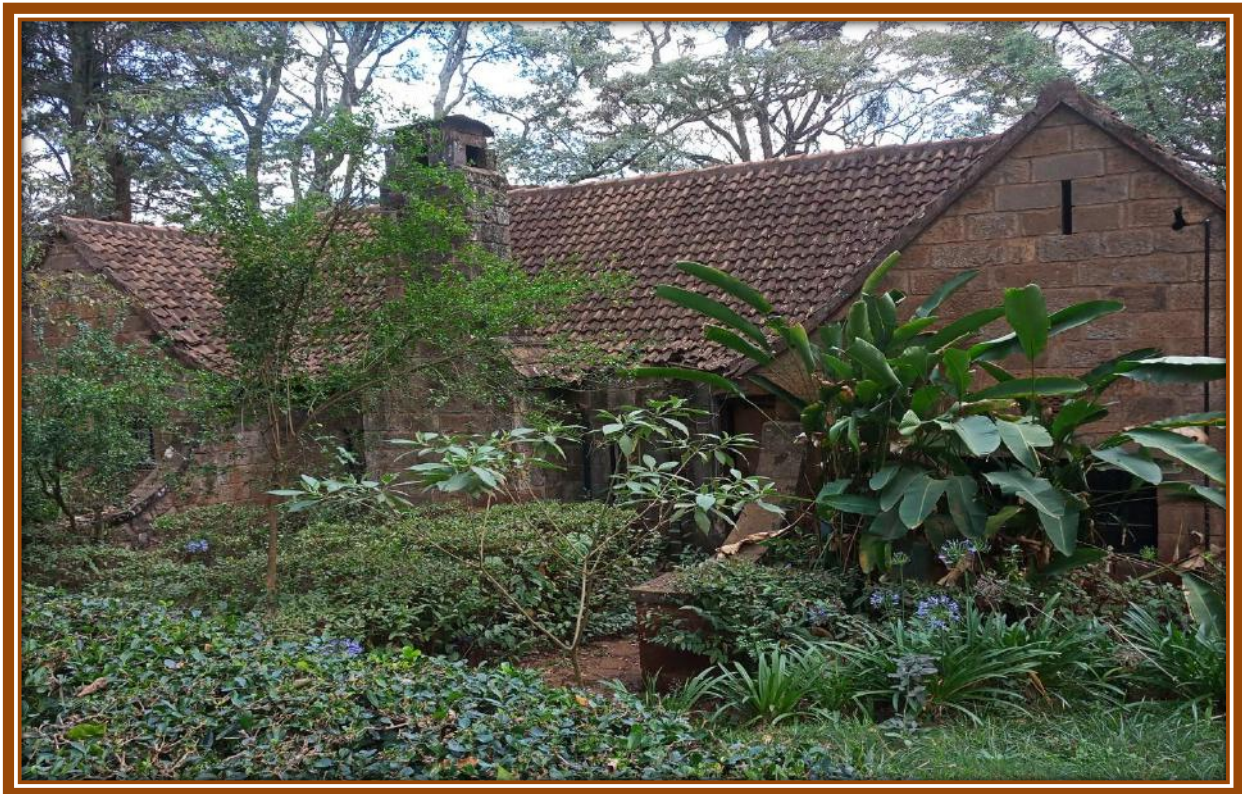
Picture 2: The long existing bungalow on the site, earmarked for demolition, on the project's commencement.
