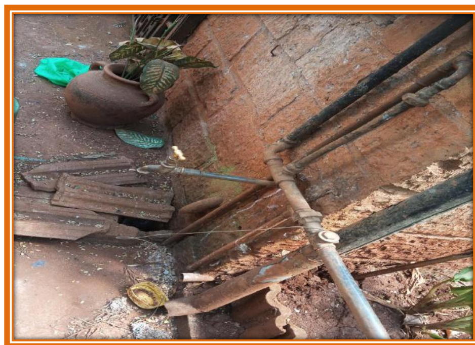
Picture 15: Existing NWC/SC's connections within the site, likely to be rerouted to allow for the impending construction works.
