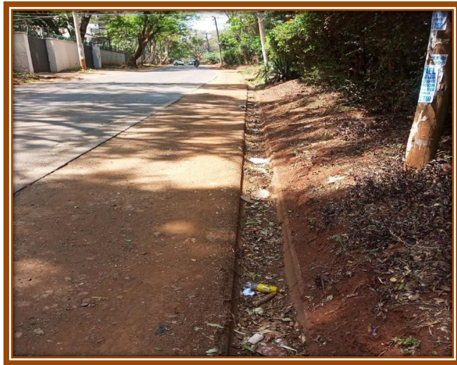
Picture 13: Clogged and unattended storm-drainage channel, along Eldama Ravine road, to which the project's will be directed.
