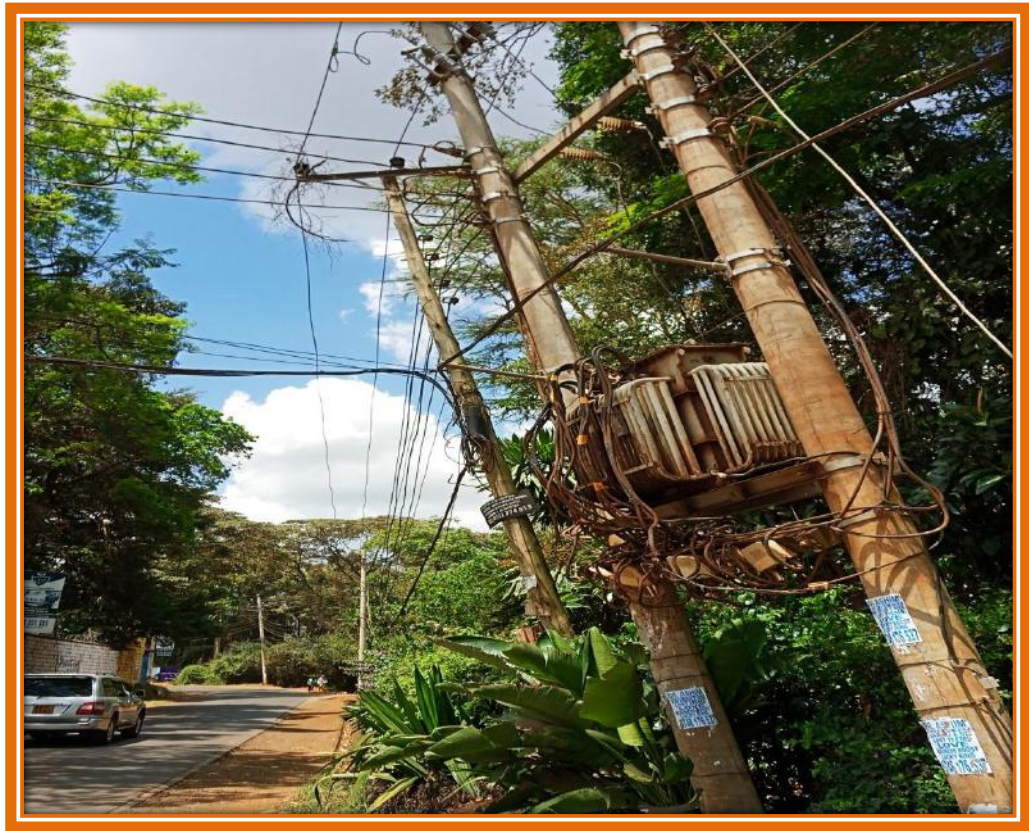
Picture 14: Reliable Power line within the area, already within the site and likely to be rerouted to allow for the construction's progress.
