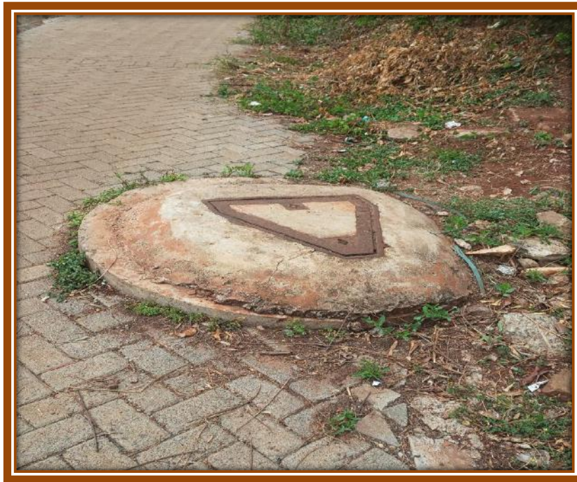
Picture 9: An existing sewer man-hole along Ring Road Westlands, about 160 metres away, to which the site's lines will be connected.
