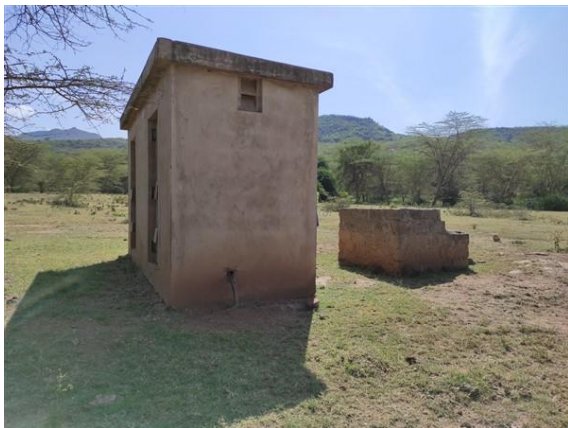
Plate 6-3: Nonproductive borehole and pump house (0° 24' 29.00"S 36°15'21.37"E)
