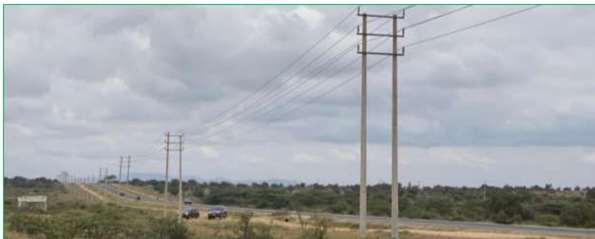
Figure 13: Reticulated power supply lines near the proposed project site (Source: Site visit, July 2021).
