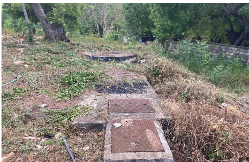
Plate 8 Existing manholes for the Septic tank & soakpit system at project site to be decommissioned
