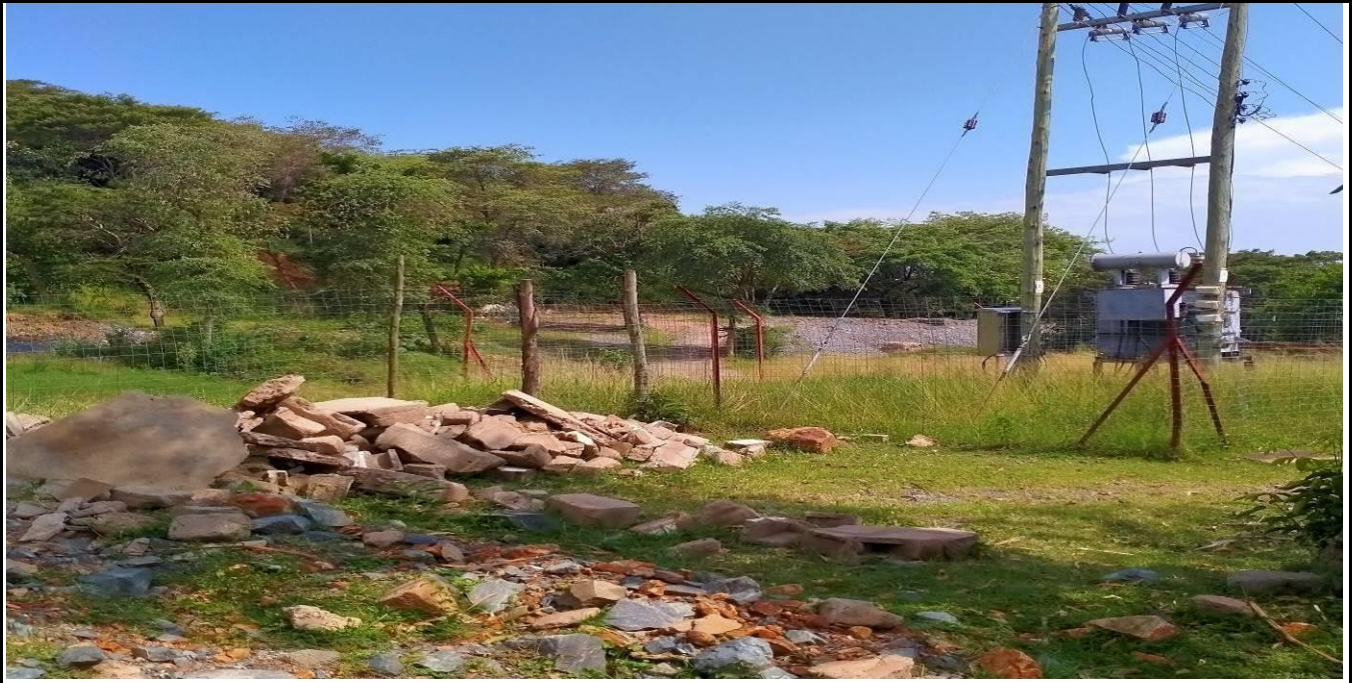
Plate 2.3: Proposed mines in the background and an electricity step down transformer at the proposed site
