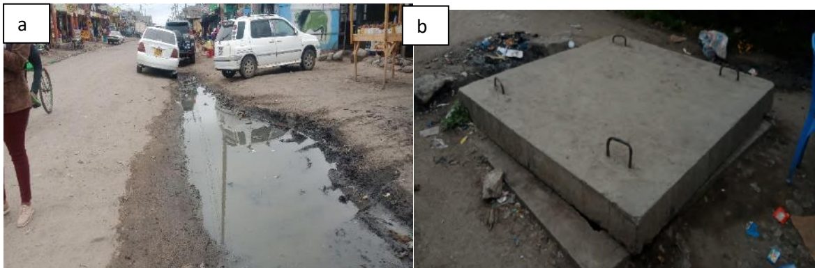
Plate 2: a) Poor drainage at Isinya town b) storm water drainage at Isinya town to be replaced
