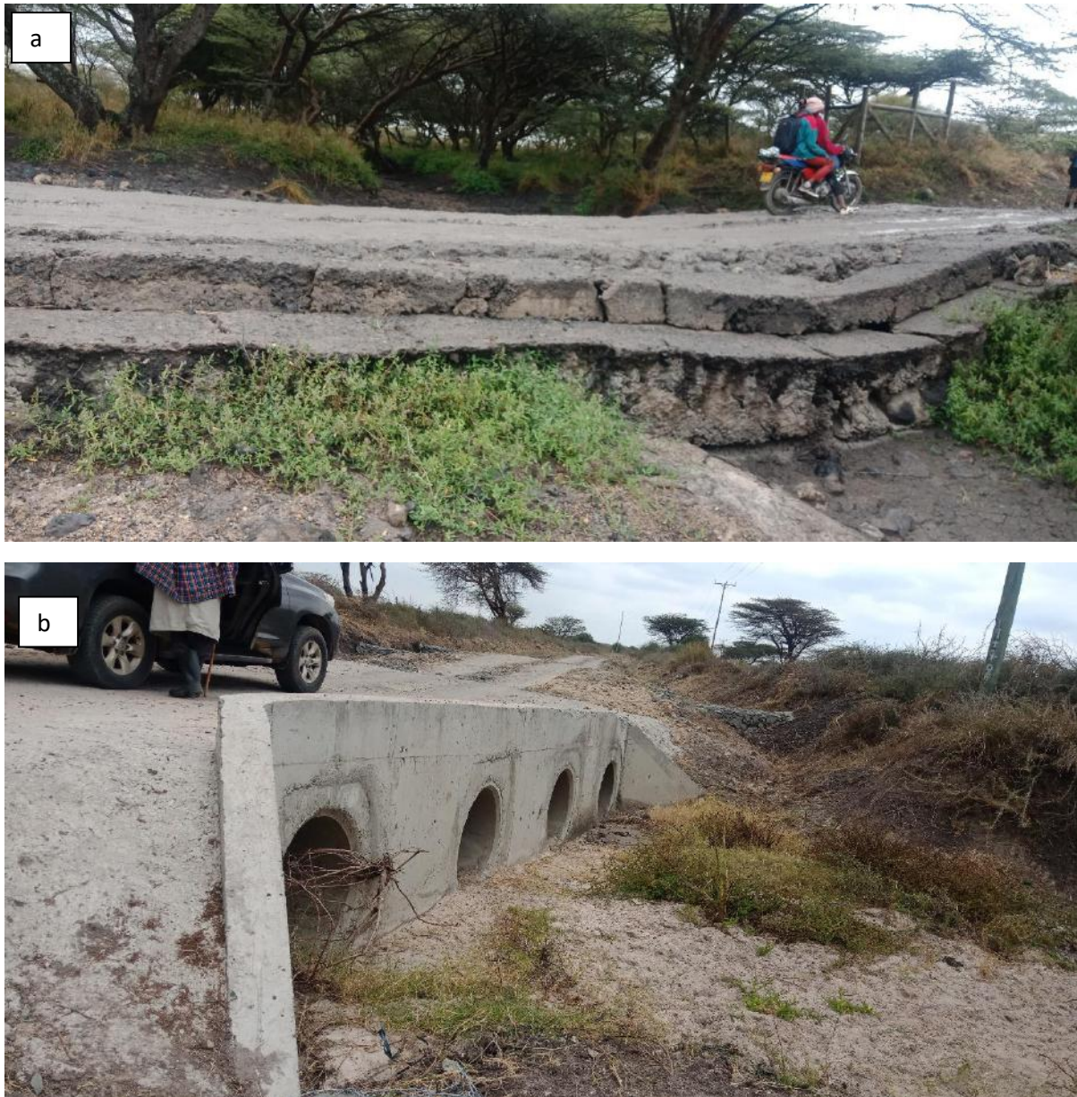
Plate 1: Sample bridges that will be replaced during construction (a) drift at Km 10 b) 4-cell pipe culverts at Km 23
