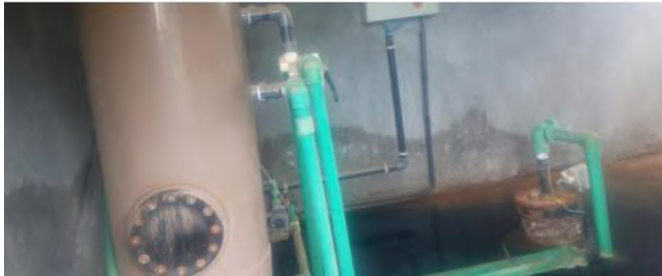
Figure 4-6: Existing on-Site Wastewater Mini-Treatment
