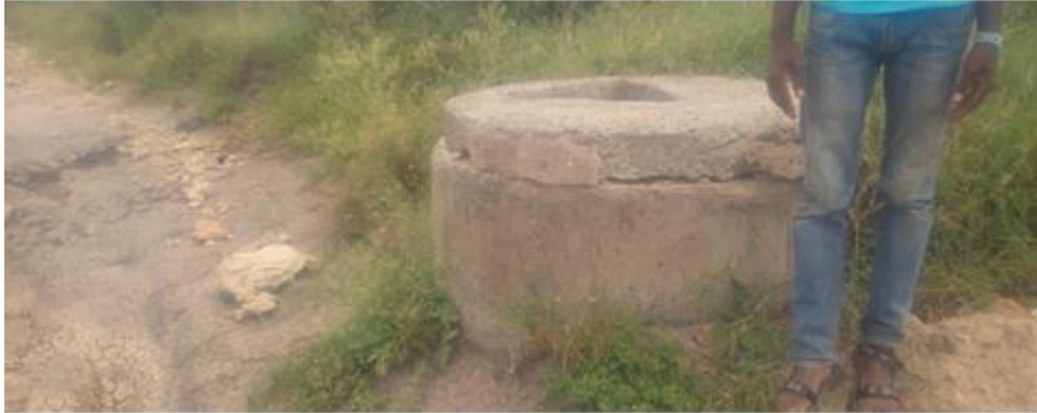
Figure 4-7: Conventional Sewer Manhole along the 18m Road
