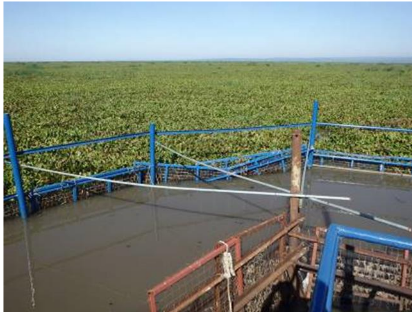
Figure 3.2 Existing water hyacinth barrier at Dunga intake
