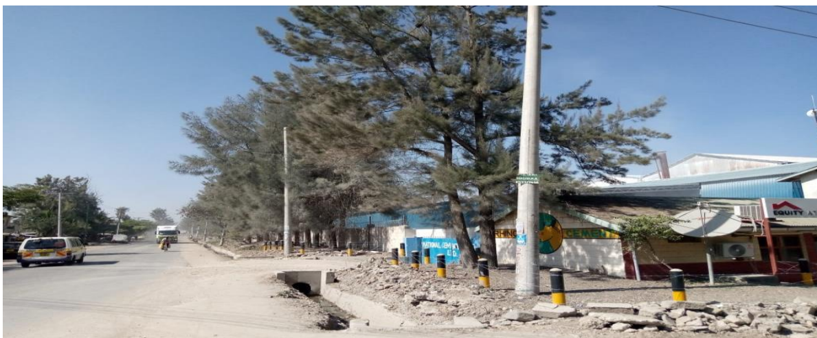
Figure 5-2: Drainage System Erected by the Plant
