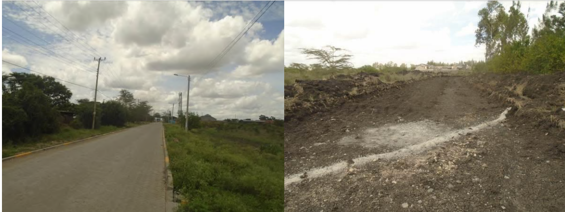
Plate 2: Cabro covered road section leading to Swiss Lounge and a section of the Access Road to the Project site
