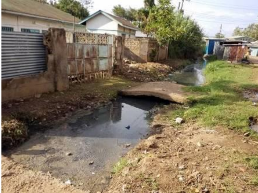
Plate 9: Raw sewer released into storm water drainage system
