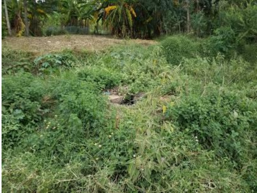
Plate 6: Manhole missing cover along Nyalenda ponds line
