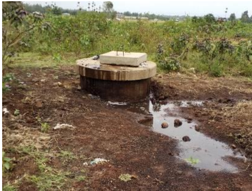
Plate 3: Blocked manhole within the line releasing raw sewage
