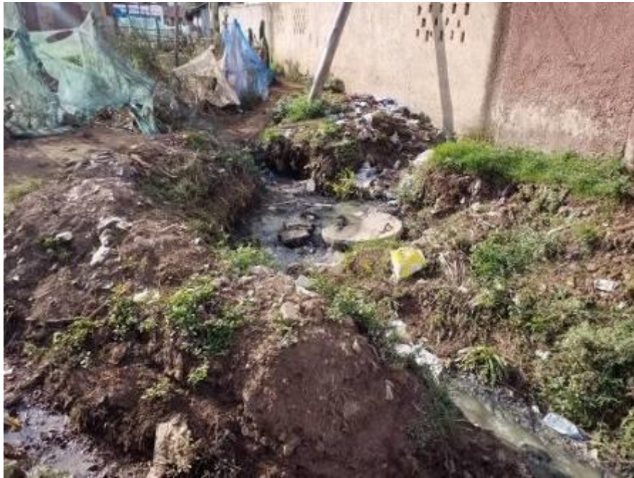
Plate 10: Blocked manhole chambers within project area
