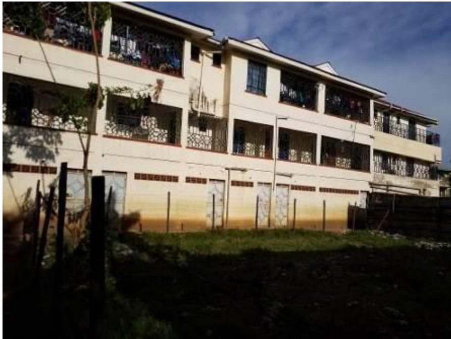
Plate 8: Building constructed on top of sewer line in Migosi area
