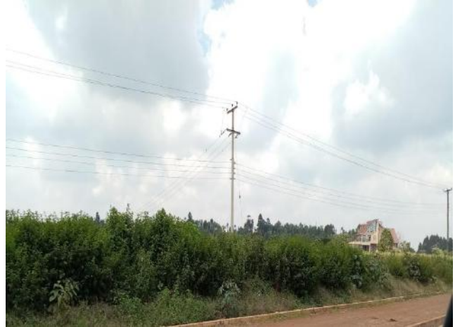
KPLC Electricity line within Migaa
