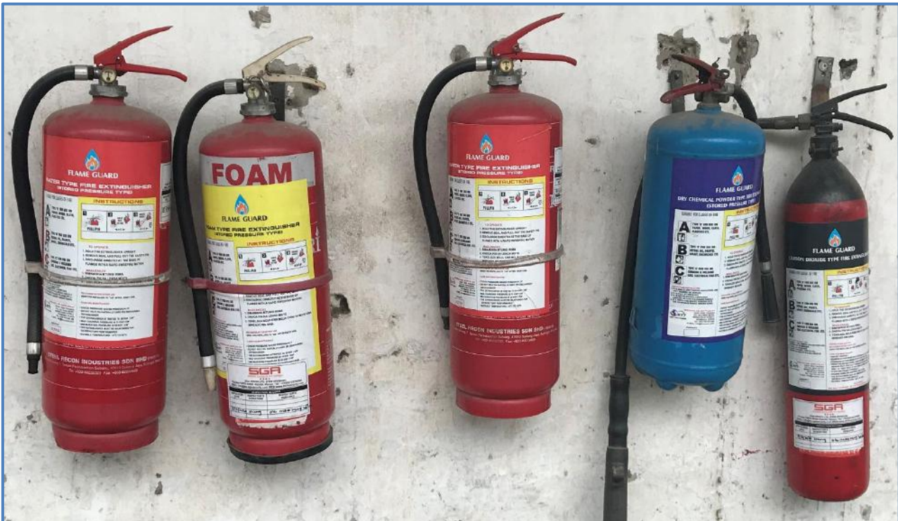
Figure 11: Existing fire extinguishers located at strategic areas of Kilindini Warehouses Limited facility (Source: Site visit, March 2020).
