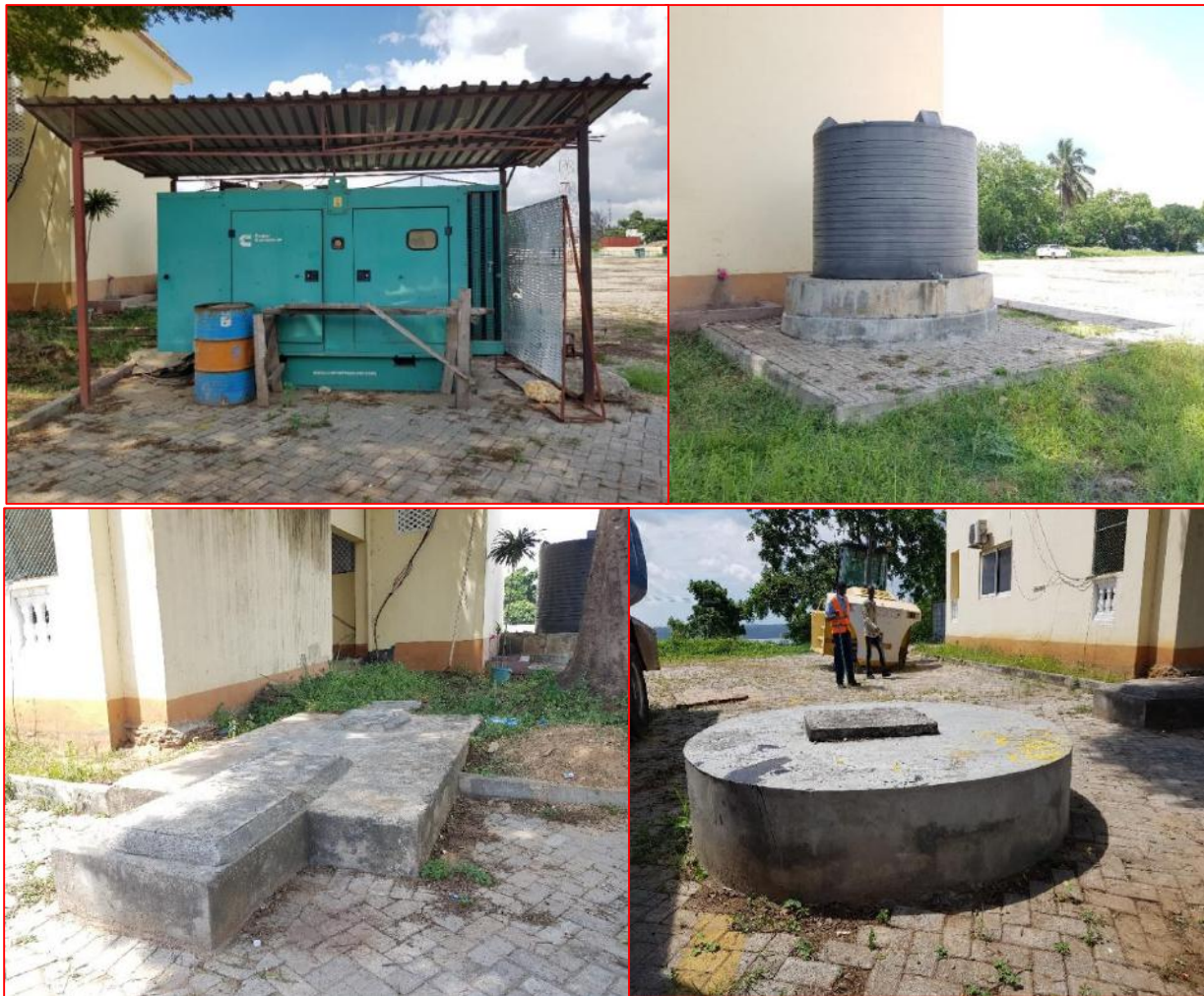
Figure 6: A section of the project site showing some of existing supporting infrastructure (Source: Site visit, November 2020).
