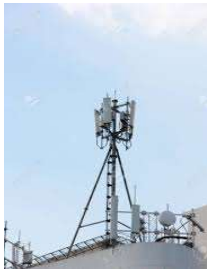
Plate 1: Photo of a Typical Rooftop BTS.
