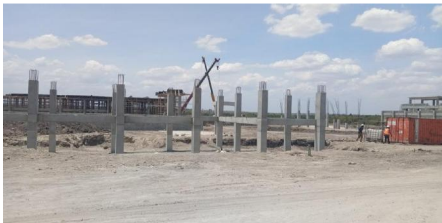
Ongoing Construction works of domestic & industrial waste water treatment nearby approximately 4km away from proposed site of Boredo Supplies Ltd
