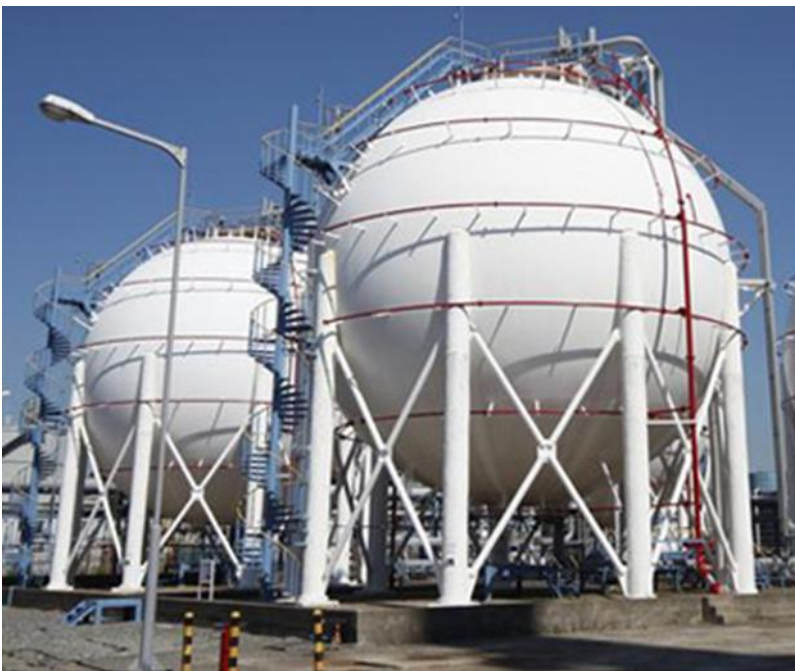
Fig 7: Above ground Spherical LPG pressure storage tanks
