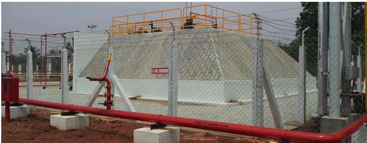
Fig 9: Concreted Mounded LPG Bullet Tank
