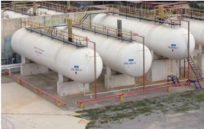
Fig 8: Above Ground Open Bullet Tanks
