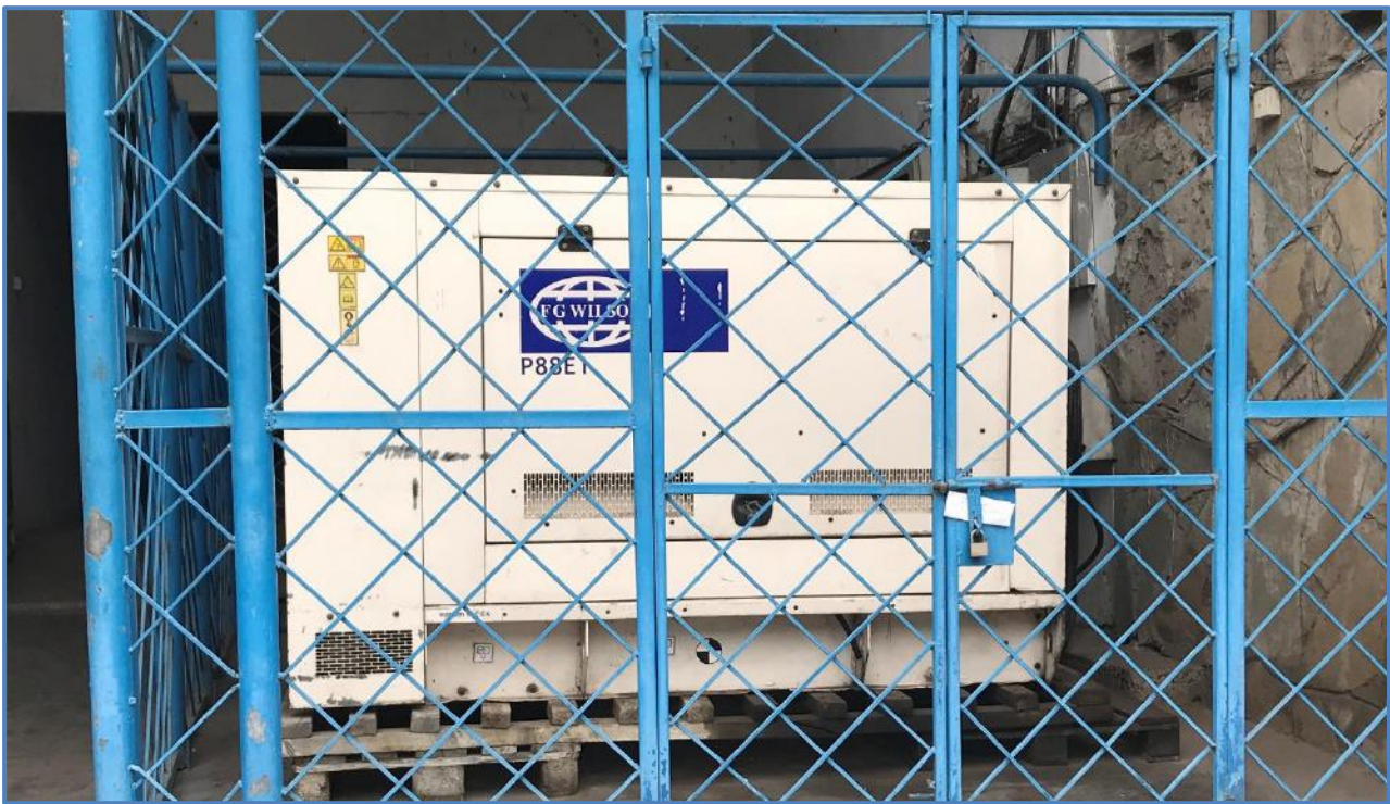
Figure 10: A standby generator at Kilindini Warehouses Limited facility (Source: Site visit, March 2020).
