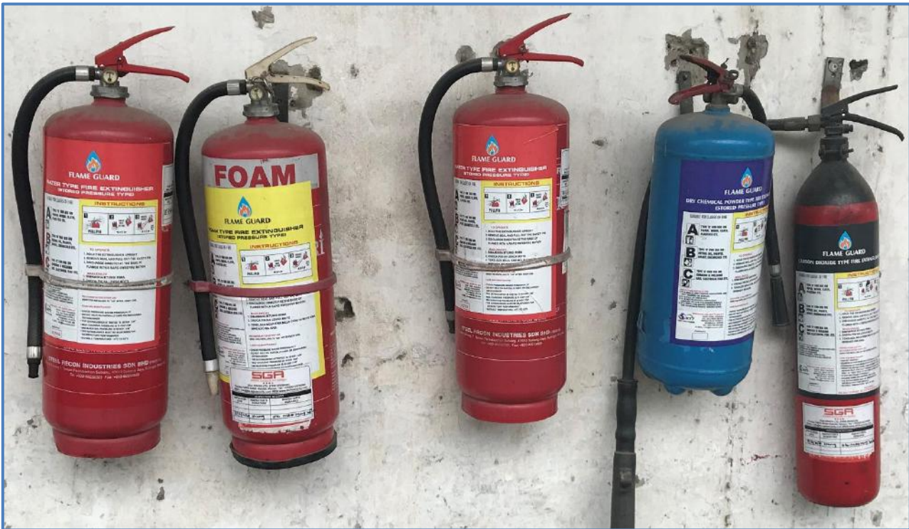
Figure 11: Existing fire extinguishers located at strategic areas of Kilindini Warehouses Limited facility (Source: Site visit, March 2020).
